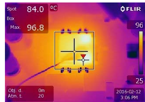
Fig. 7. Thermal Image with 3 Hot Spots
